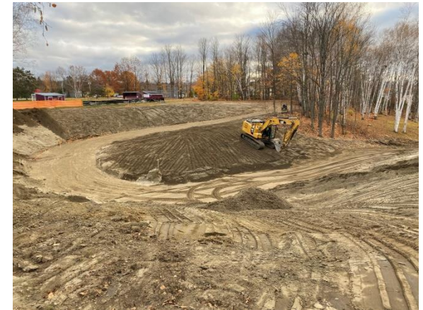
Work in progress on the Prouty Beach Connector Trail, which was completed and dedicated in the fall of 2021, and connects the seven-mile recreation corridor between downtown Newport and the Canadian border.
